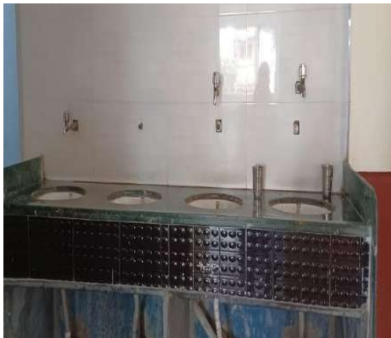
Provision of Safe drinking water and purifier facility
