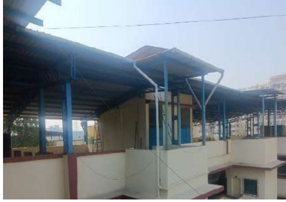
Water Tank on the roof top
