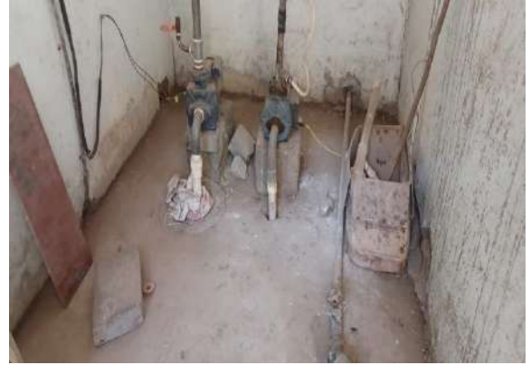
Two water connections and water meter in campus
