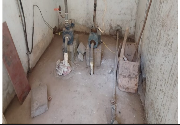
Two water connections and water meter in campus
