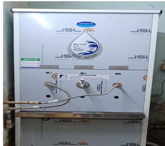
Water purifier facility
