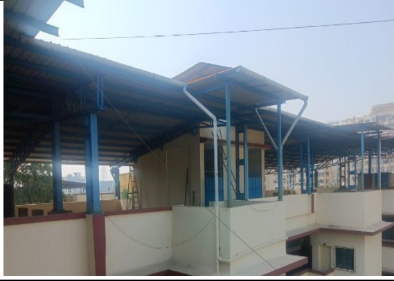
Water Tank on the roof top
