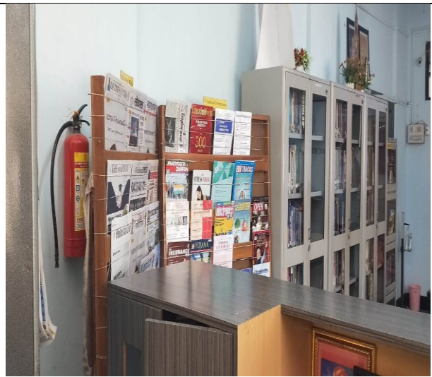
Installed Fire Extinguisher inside college library
