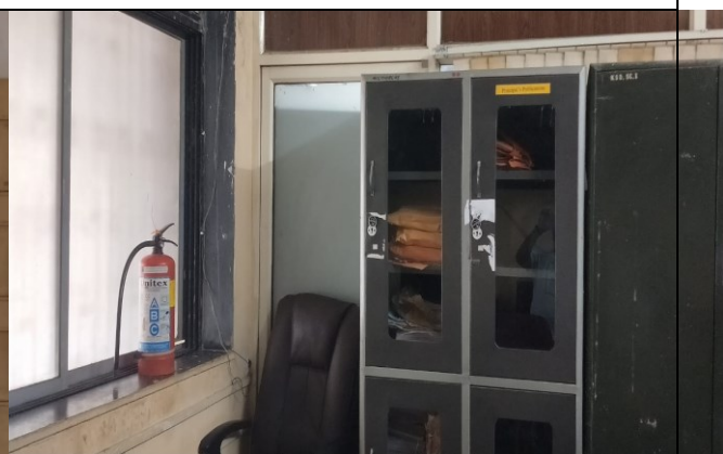
Fire Extinguisher in College Office
