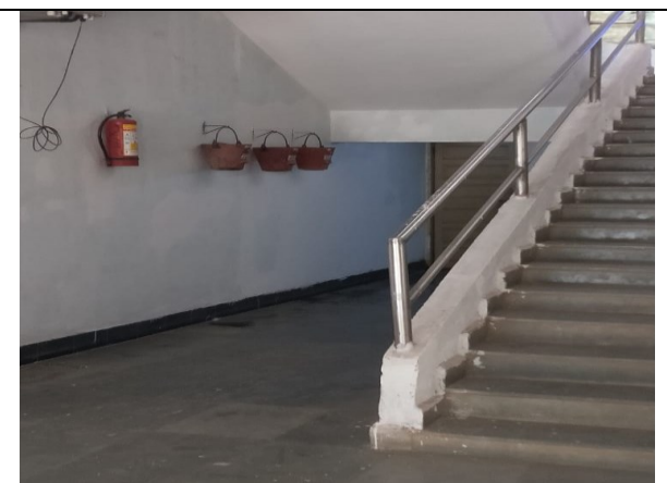
Fire Extinguisher in Staircase
